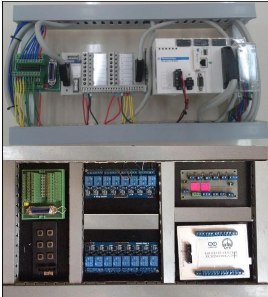
Figura 72: Tablero de control TC002
