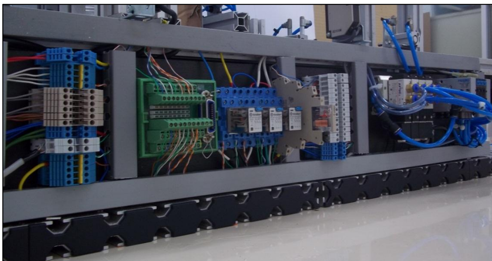
Figura 73: Tablero de control TC001
