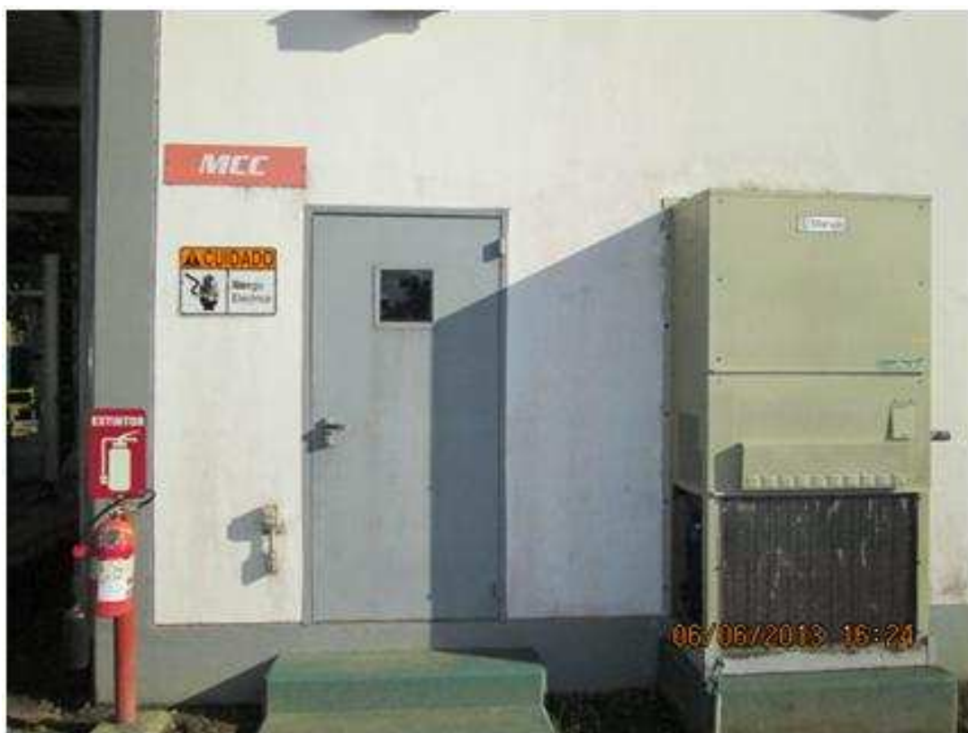
Figura 2.44. MCC (Motor Control Center)
