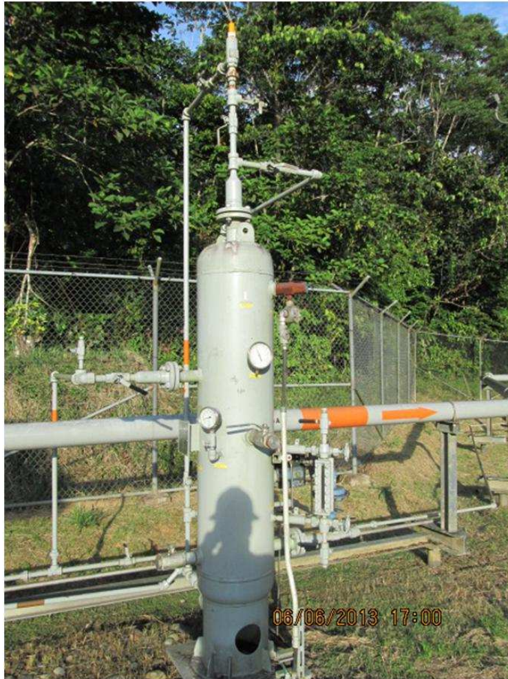
Figura 2.38. Scrubber de Gas
