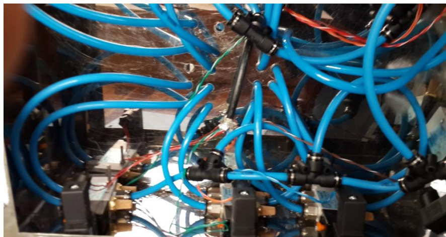
Figura 4.64. Electroválvulas instaladas (Loaiza, 2014)
