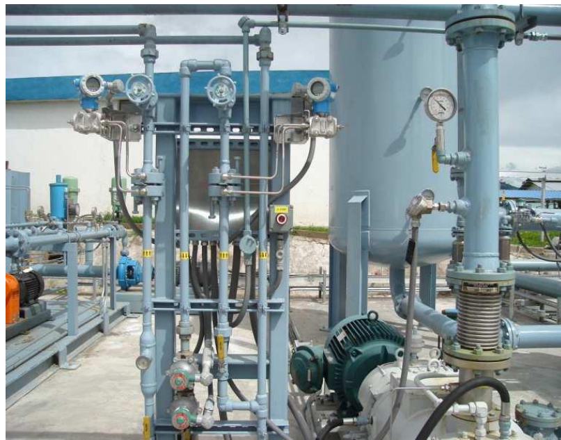
Figura N° 2. 29 Coolant Flow Transmitters
