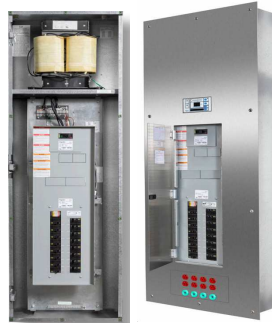
Figura 51. Tablero de aislamiento hospitalario IT. (BENDER, 2020)
