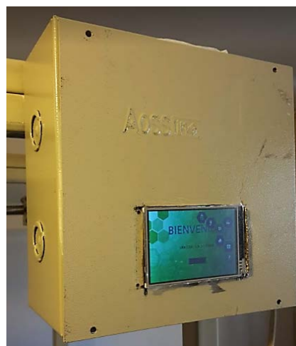
Figura 40. Panel de control
