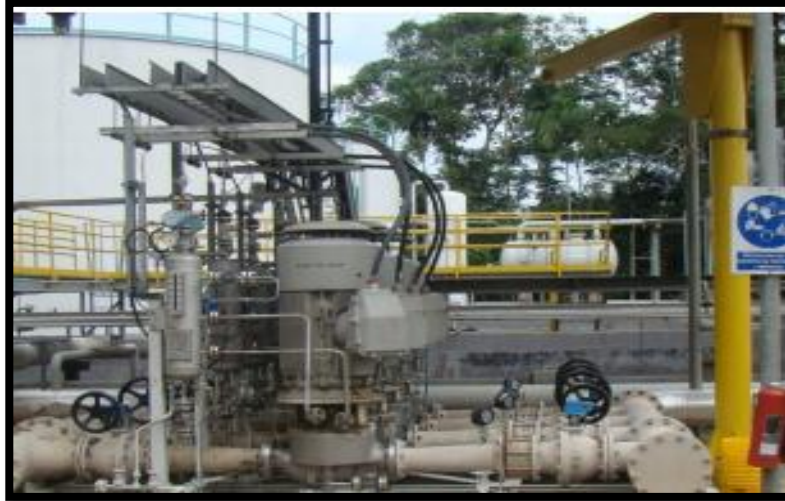
Figura 14. Bombas Booster A/B/C (AGIP OIL)
